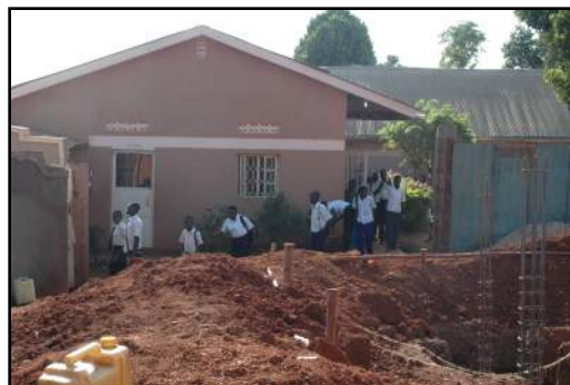
During construction, students still attend school in the other classroom blocks Alice and Mtaala constructed.
