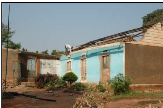
To make way for the new school building, demolition begins on Alice's former home, the house she had turned into a school for needy students.
